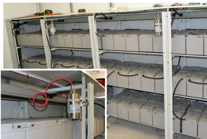
FP 100 FirePro Generators within Battery Cabinet Insert shows linear heat detection cable
